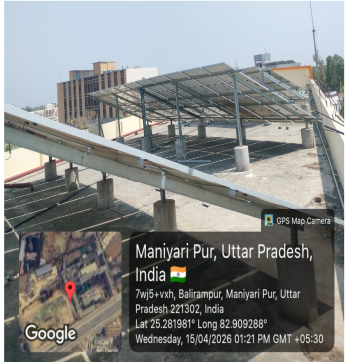
50 Kw Solar Pannel
